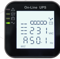
Module Control Panel
